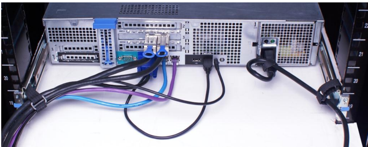
Figure 12. Cabling a system installed in static rails
